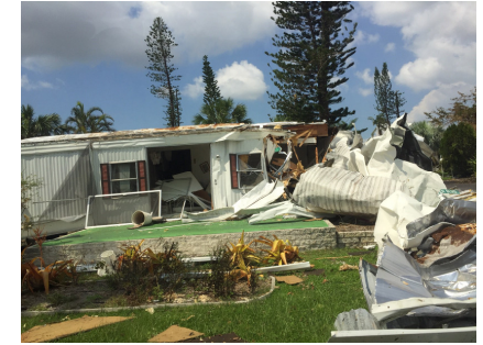
Home destroyed in Florida. FEMA News Photo
